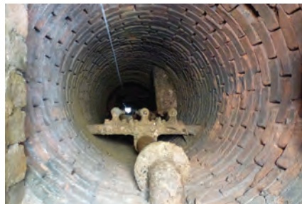
Looking inside an old, hand dug water well. Many historic boreholes started life as a hand dug water well and were later deepened by drilling.
